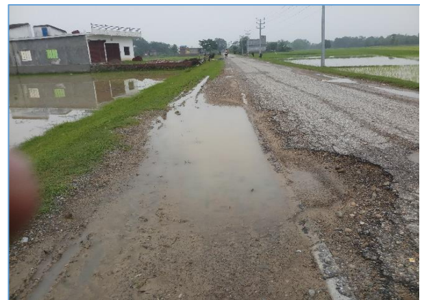
Figure No 5.2: Urban Road Condition at Ward 6
